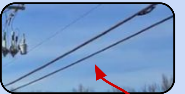
Overhead Power Lines
